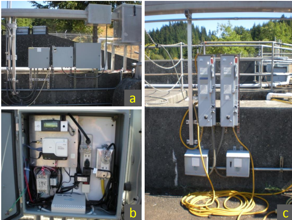
Figure A6. System controls at electrical box (a-b) and pump panels (c) for Washington Shore AWS LPS.
