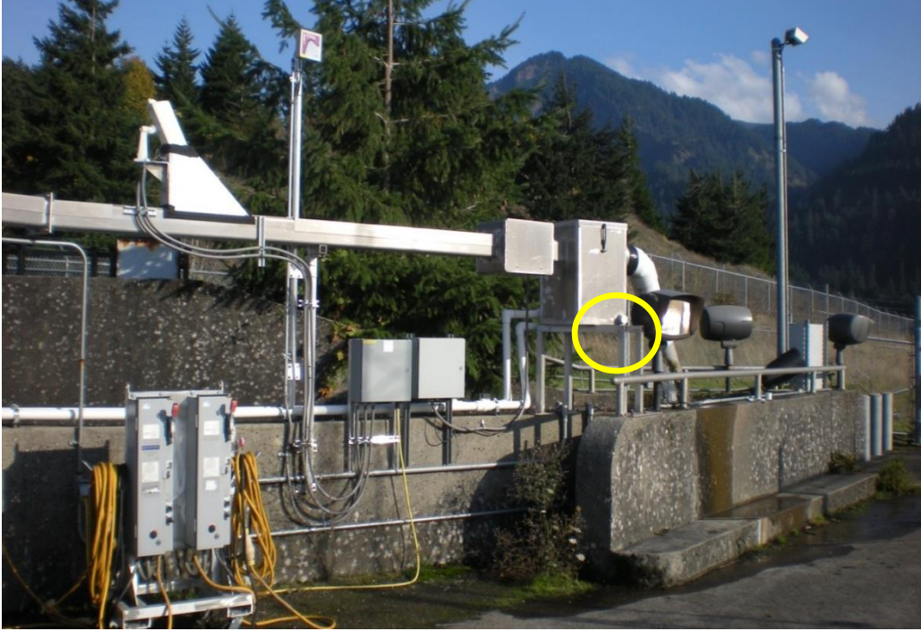
Figure A4. Discharge valve at Washington Shore AWS LPS upwelling box.
