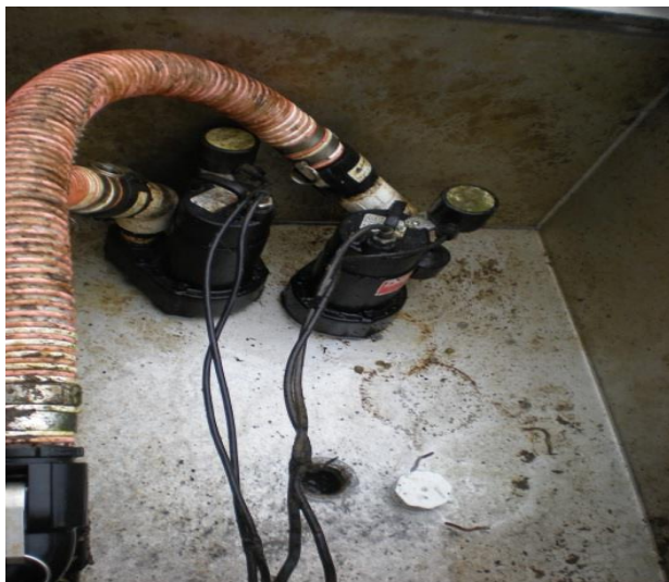
Figure C7. Upstream transition pond showing pumps and unplugged drain in reservoir at Cascades Island LPS.
